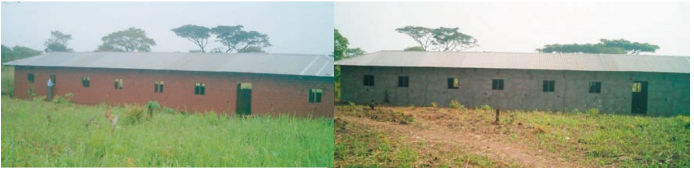
(L) Health Center walls are up to the roof, (R) and plastered with cement mix to protect them against rain.
