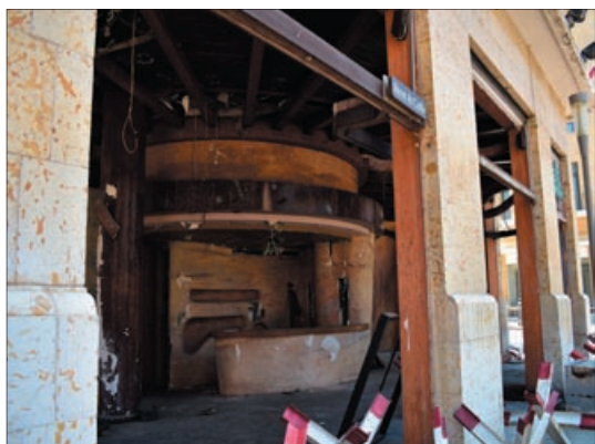
Many shop windows are still gone after the explosion in the harbour of Beirut in 2020
